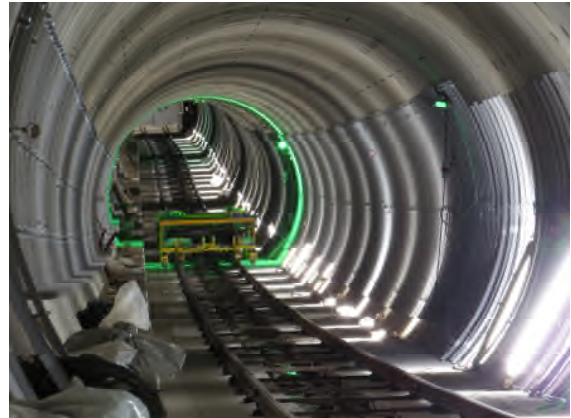
Connection of the left-hand track to the existing metro line (photo Metrostav a.s.)
